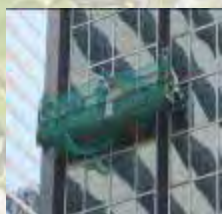
Refurbishment works relating to curtain wall at Immigration Tower implemented by ArchSD
