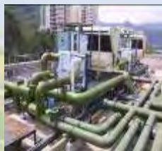
Replacement of air-cooled chillers by binary ice chillers at Mui Wo GO
