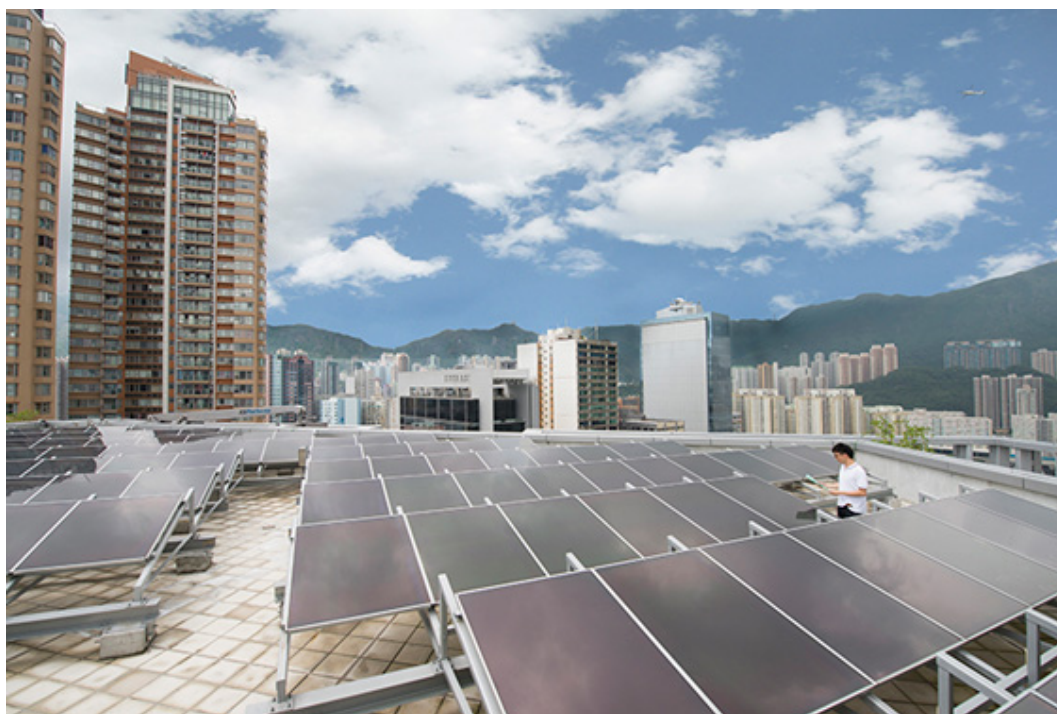
PV Panels installed at Trade and Industry Tower
