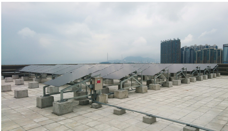
PV panels at WKGO
