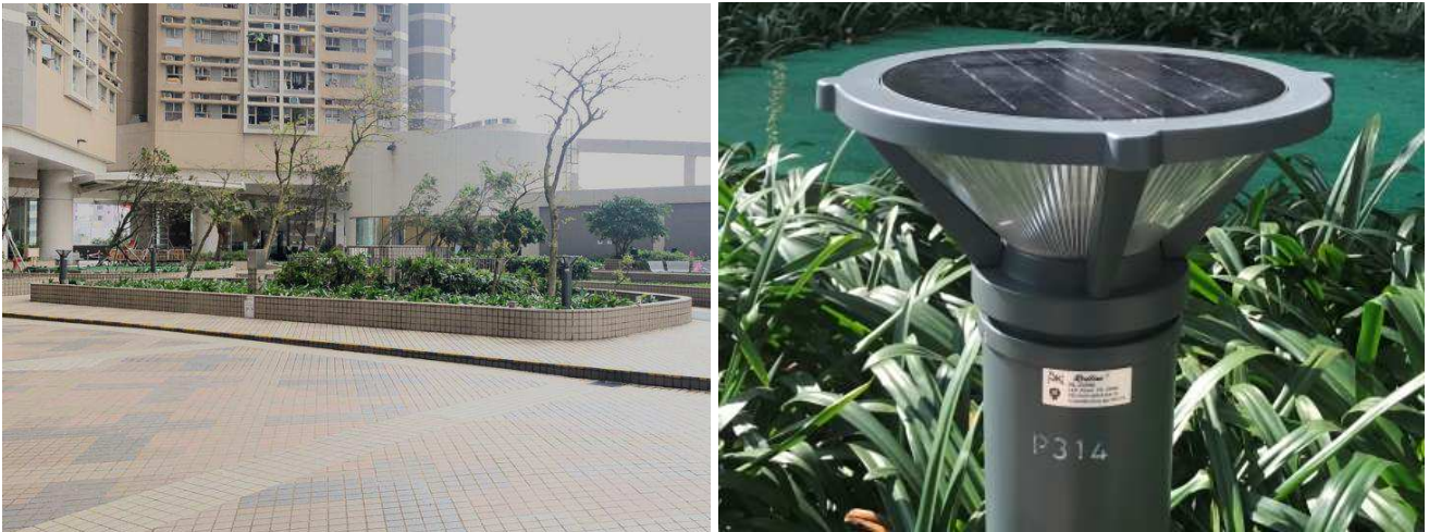
Solar bollard installed at Shun Lee Disciplined Services Quarters
