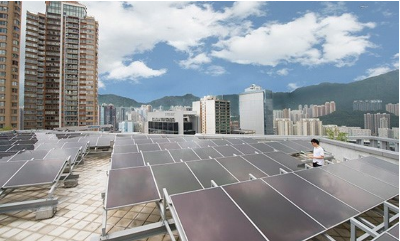
PV Panels at Trade and Industry Tower
