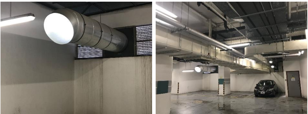
Daylight suntube at Shun Lee Disciplined Services Quarters
