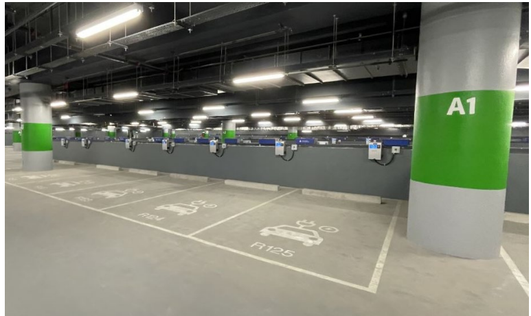
EV chargers at Heung Yuen Wai Boundary Control Point public car park
