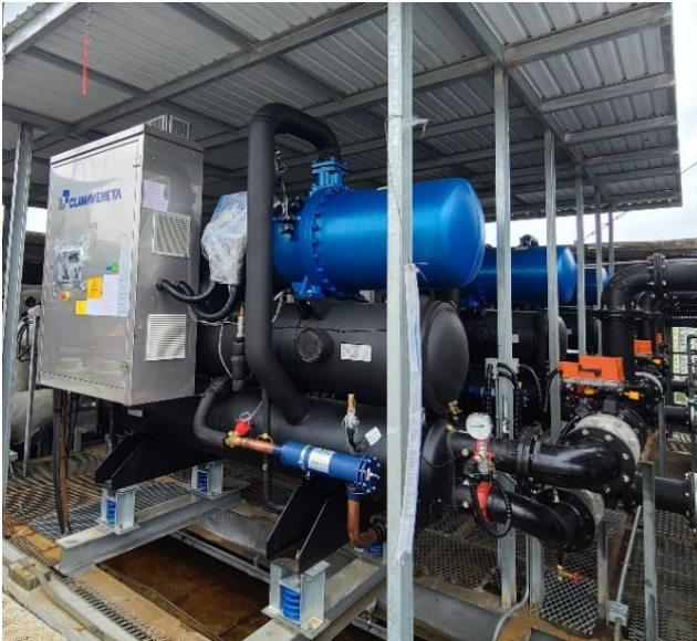
Water-cooled screw chiller with variable speed drive replacement works at Lai Chi Kok Government Offices
