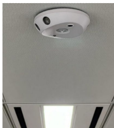
Occupancy sensor for lighting control at West Kowloon Government Offices
