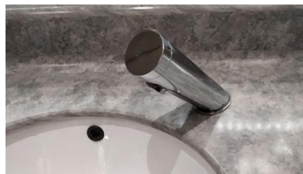
Sensor water tap in joint-user general office buildings
