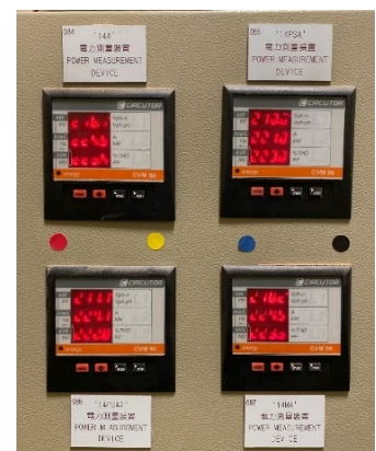
Local meter to monitor electricity consumption at Harbour Building
