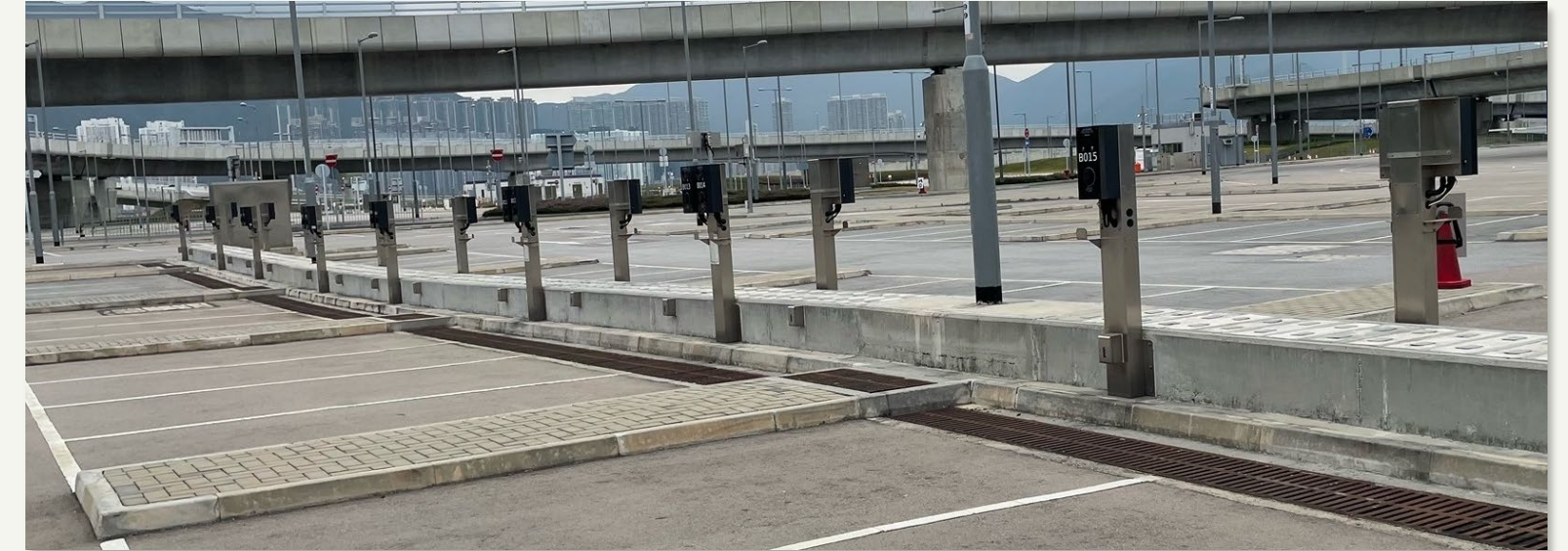
EV chargers at HZMB HKP public car park
