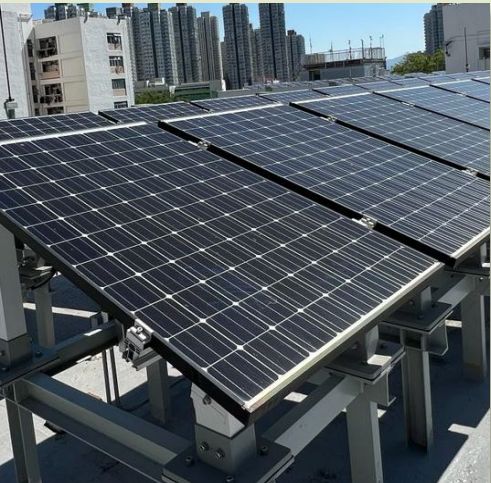
Photovoltaic panel system at Tai Po Government Offices
