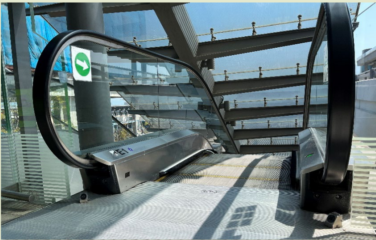
Services-on-demand escalator at HZMB HKP
