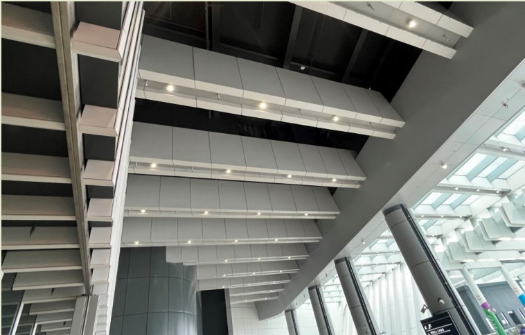
LED lightings with automatic control at Passenger Terminal Building in HYW BCP
