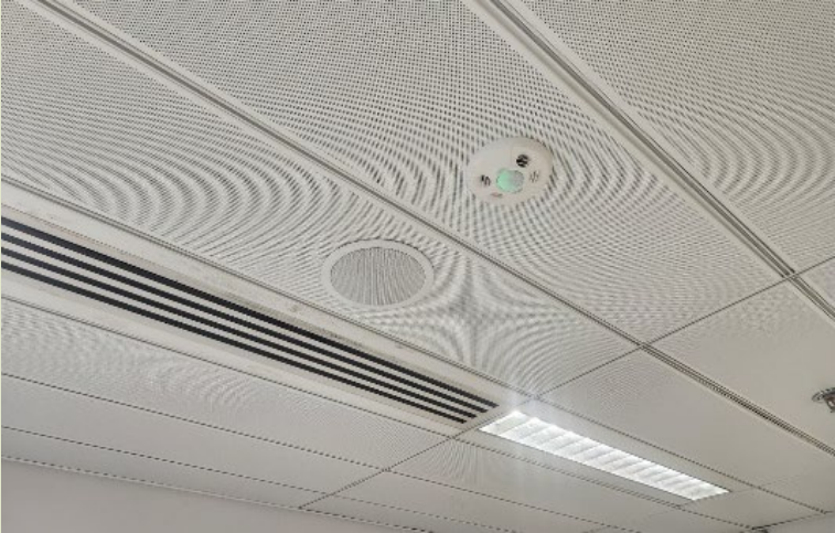
Occupancy sensor of lighting control at Trade and Industry Tower
