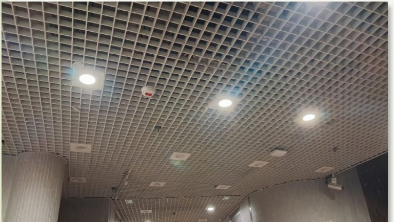
Switching off portion of lightings at Lai Chi Kok Government Offices during non-operating hours
