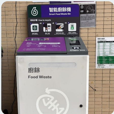
Smart Food Waste Bin at Shun Lee Disciplined Services Quarters
