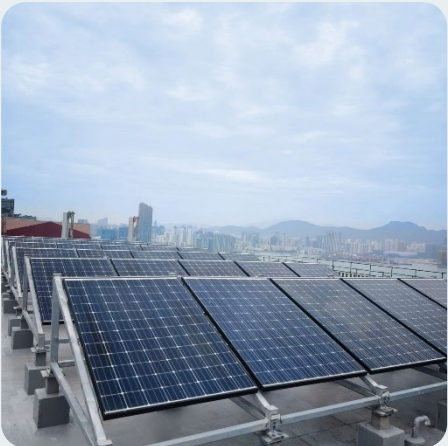
Photovoltaic panel system at North Point Government Offices
