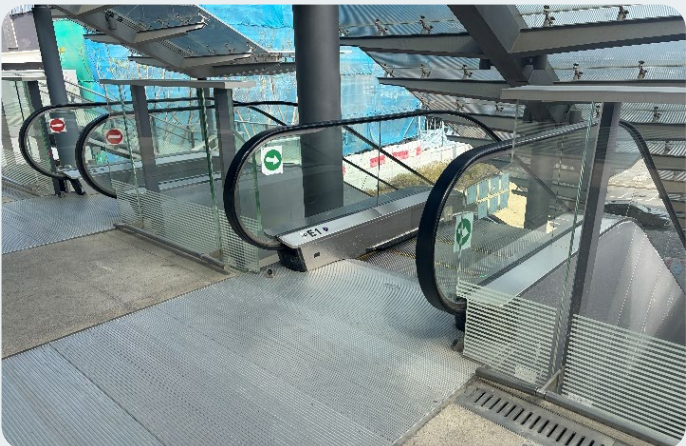
Service-on-demand escalators at HZMB HKP
