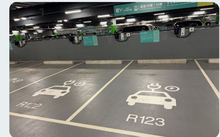
EV chargers in public carpark at HYW BCP
