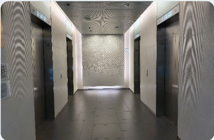
Power regenerative lifts at West Kowloon Government Offices
