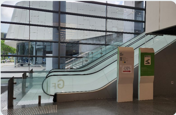
Service-on-demand escalators at Trade and Industry Tower
